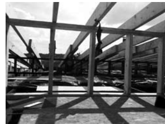
Roof repairs made to a building in Braddock, Pennsylvania. The roof needed replacing and the first stage of replacing the rafters took about 10 days with a group of 4 friends from NYC, 2009.
